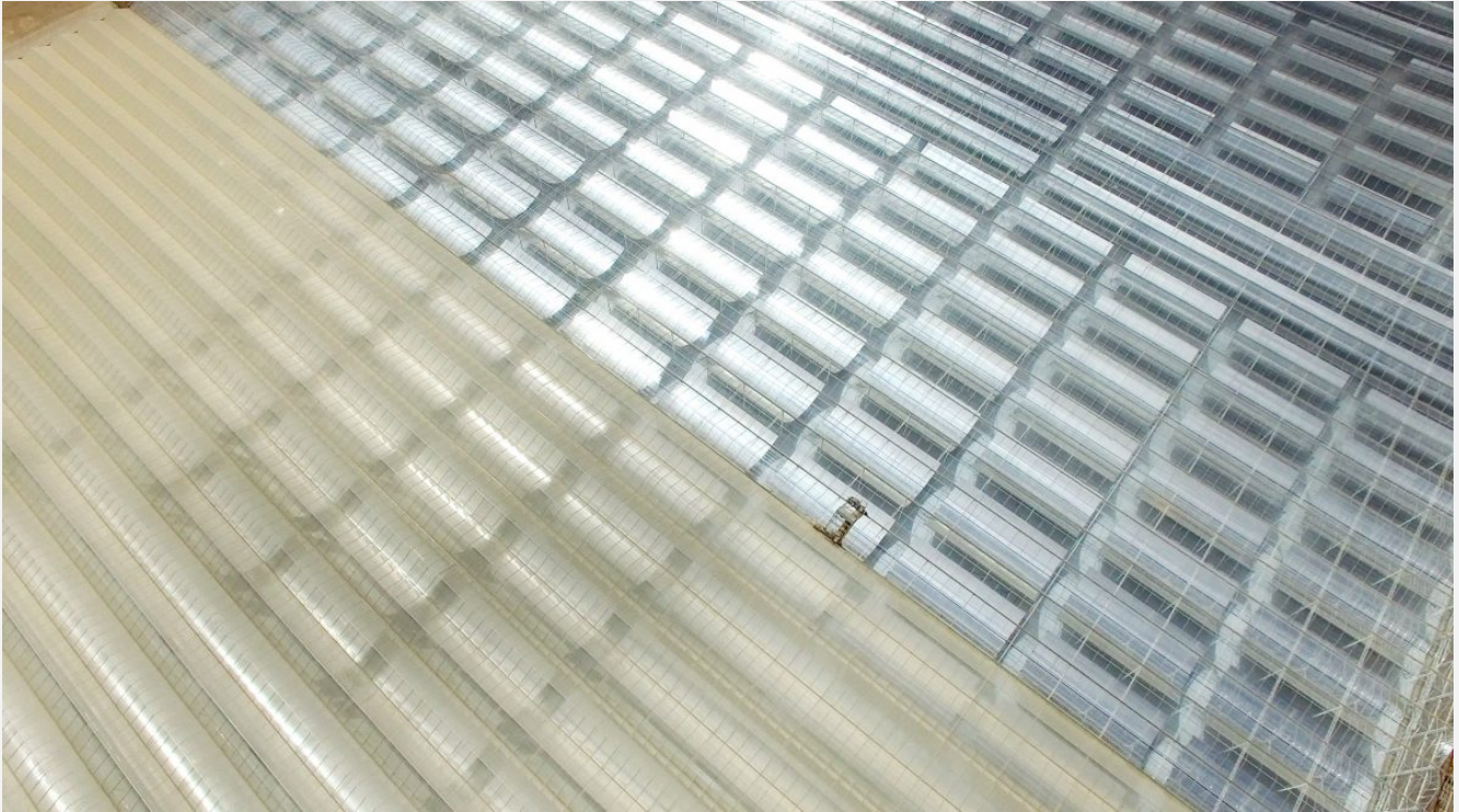
The difference between a dusty array and a clean one is clear in this photo. Note the robotic window washing machine traversing the last row of the clean part. Source: GlassPoint Solar
